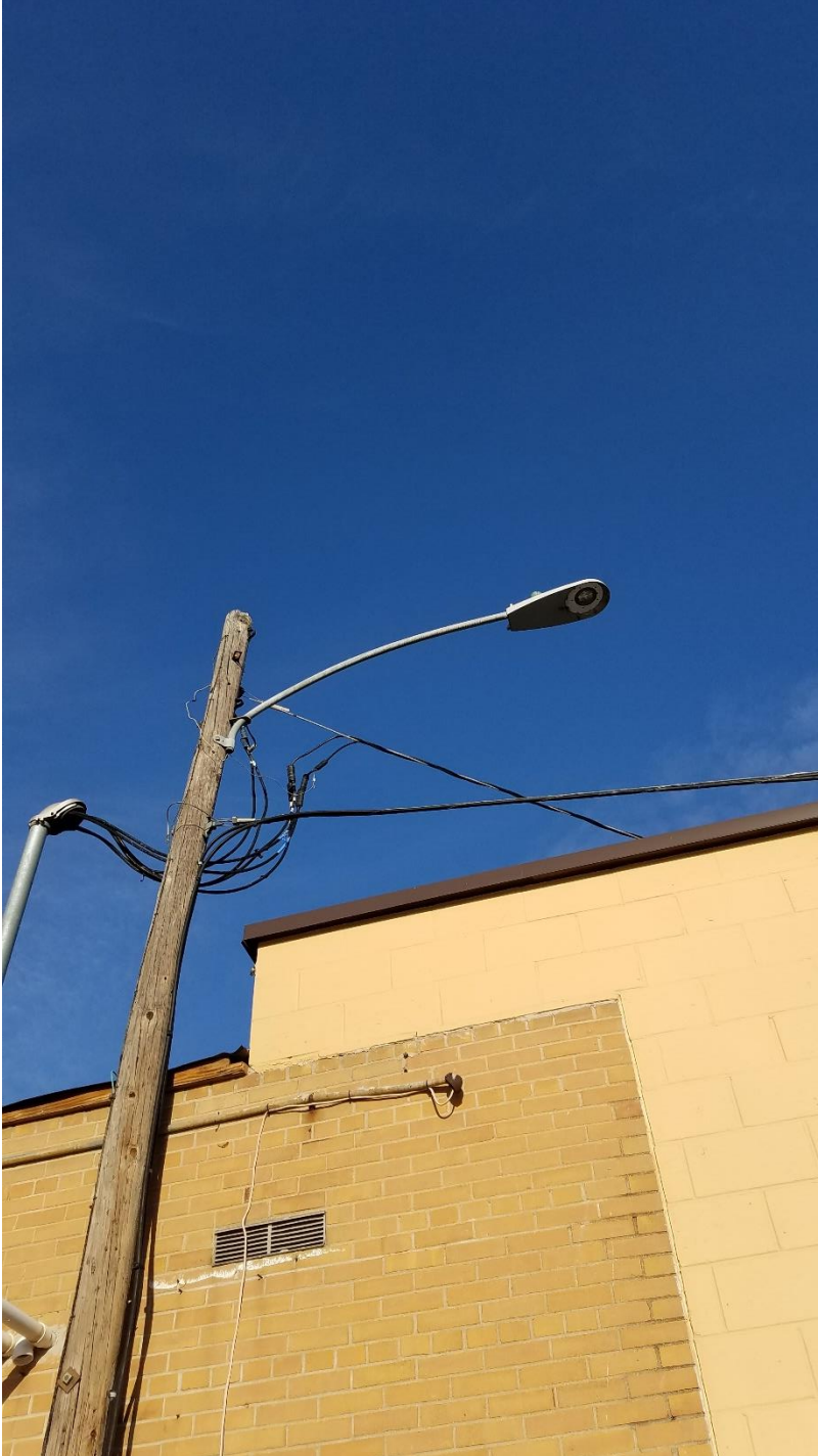
FIGURE 7 POLE MOUNTED FIXTURE AT AMBULANCE BUILDING SITE
