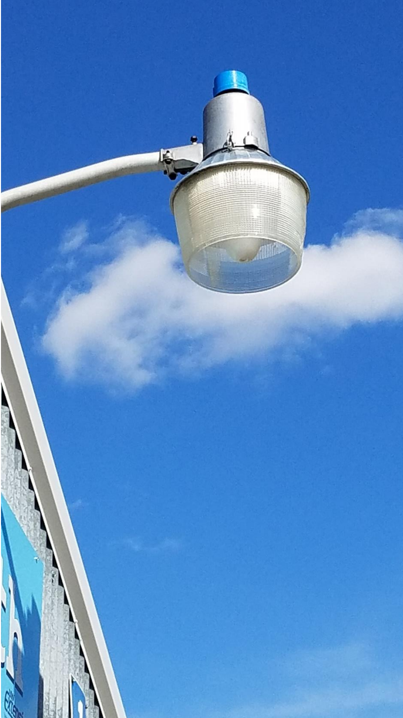
FIGURE 8 TYPICAL WALL MOUNTED YARD LIGHT AT FAIRGROUNDS SITE
