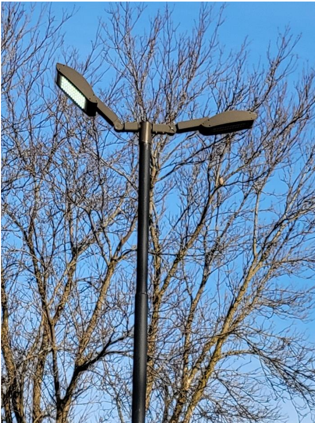
FIGURE 1 - PARKING LOT LIGHT AT CAMPUS SITE
