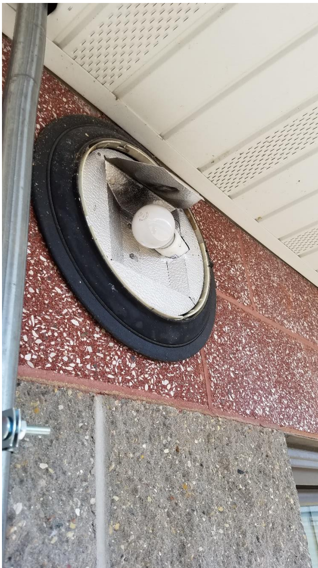
FIGURE 9 DAMAGED SCNCE ON BUILDING 2 AT FAIRGROUNDS SITE
